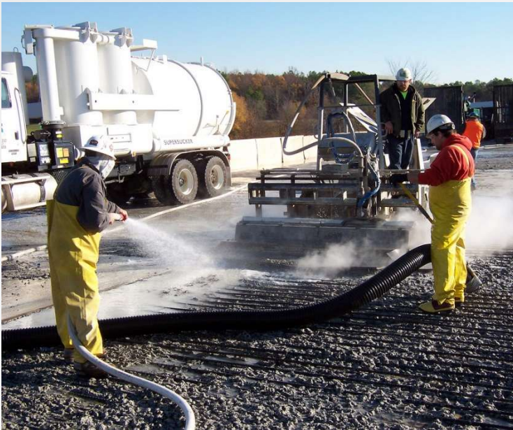
NCDOT.(2005). Hydro-demolition work on bridge deck [Digital Image]. Raleigh, NC: NCDOT Communications.
