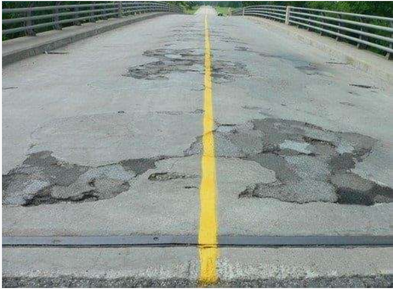
Use of Ultra-High-Performance Concrete for Bridge Deck Overlays - Scientific Figure on ResearchGate. Available from: https://www.researchgate.net/figure/Typical-examples-of-bridge-deck-deterioration_fig1_323883743 [accessed 4 Apr, 2019]
