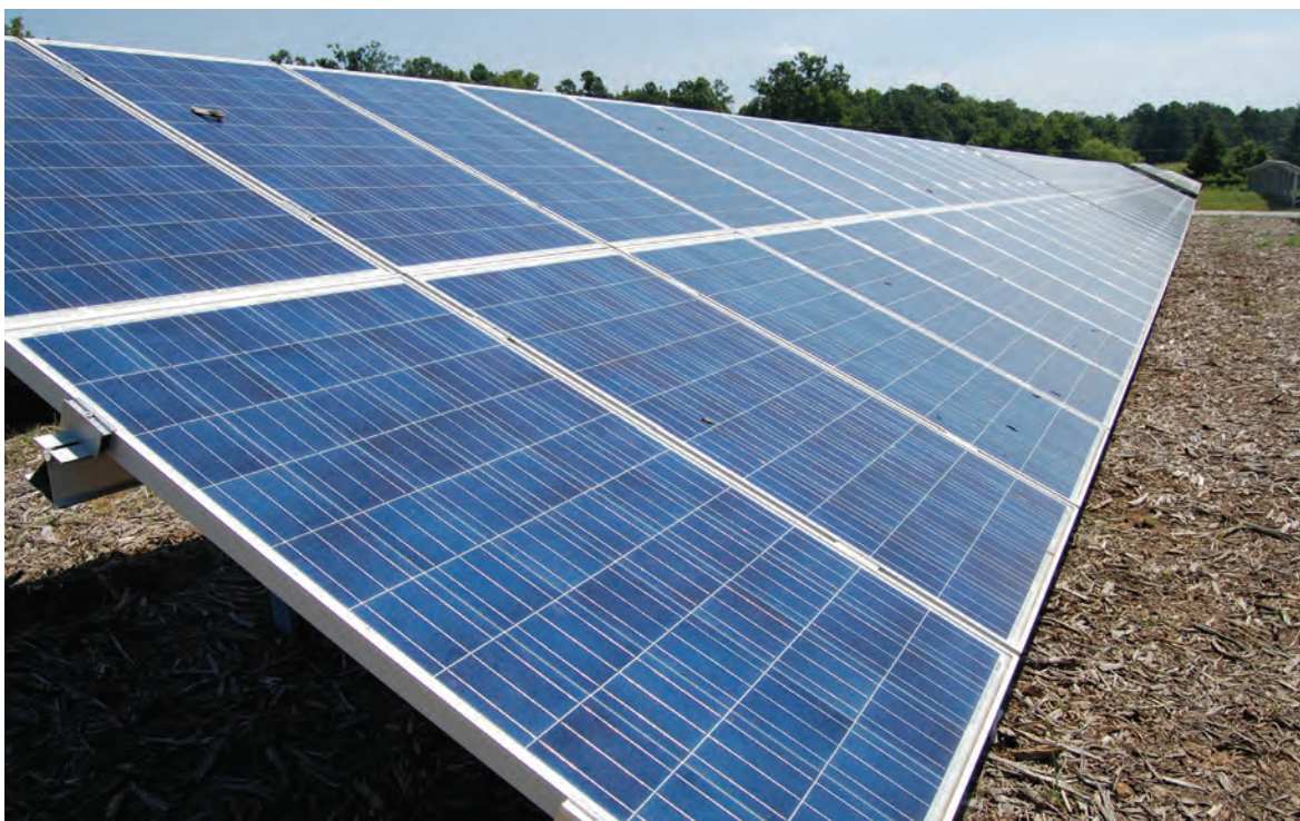
Photovoltaic panels (or modules), here on a solar farm, convert sunlight into electricity.
