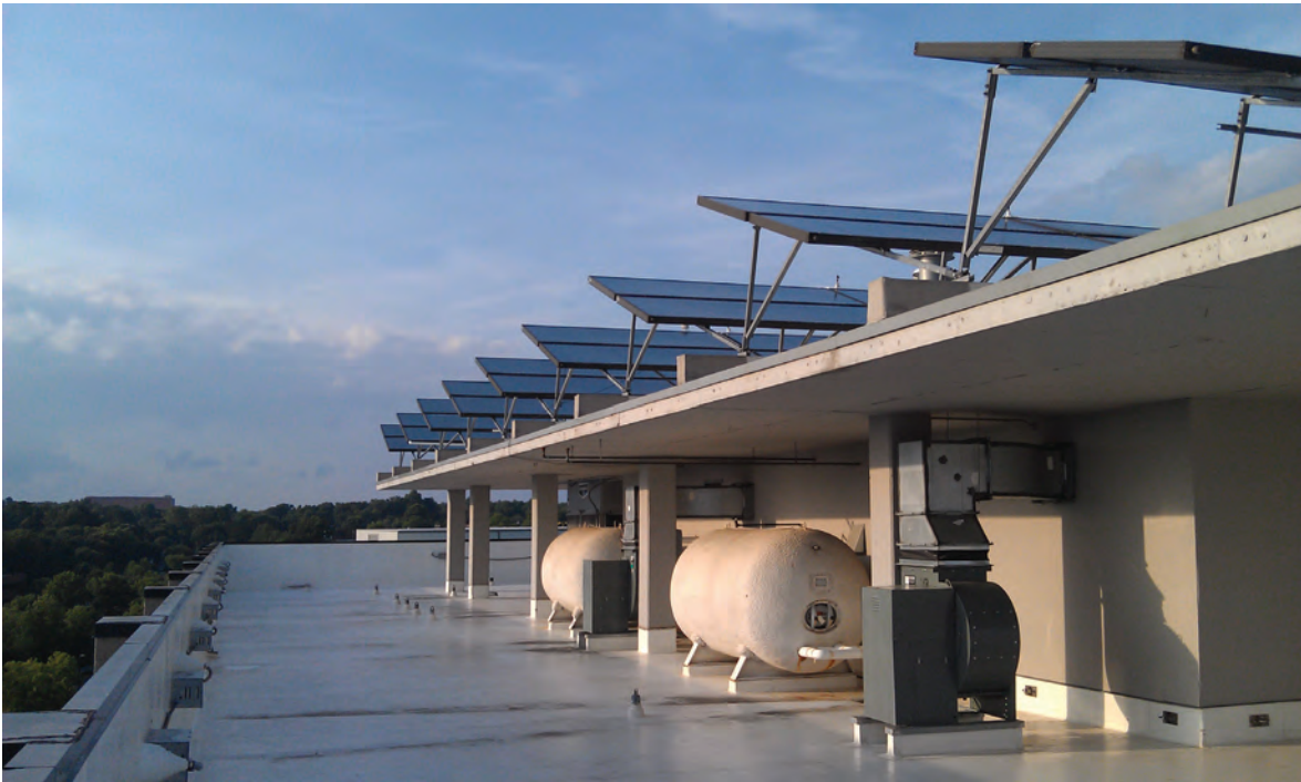
Solar thermal panels atop the Proximity Hotel in Greensboro. The hotel earned LEED® Platinum certification from the U.S. Green Building Council.
