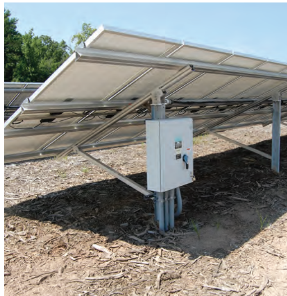
Ground-mounted PV panels.
