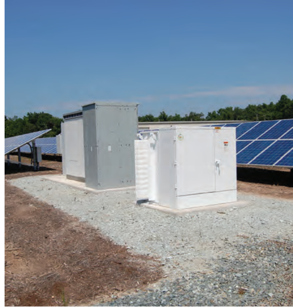
Inverters—the equipment needed to convert the current from DC to AC—create a minor amount of noise.
