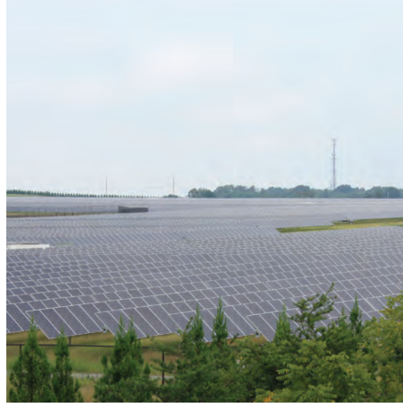
Solar farms are large-scale solar installations such as Apple's farm near Maiden, North Carolina.
