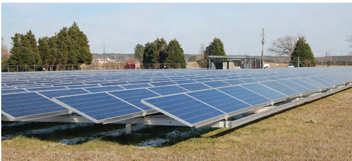
Raleigh has converted land near a wastewater treatment plant into a solar farm.
